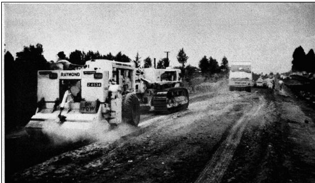
The picture above and the one at the foot of the page show the Wood preparizer at work preparing the material for the sub-base of the road prior to stabilizing.
