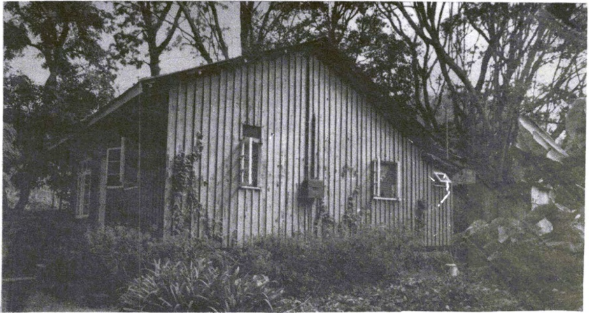
Mrs Wangio's House Falling Apart.
