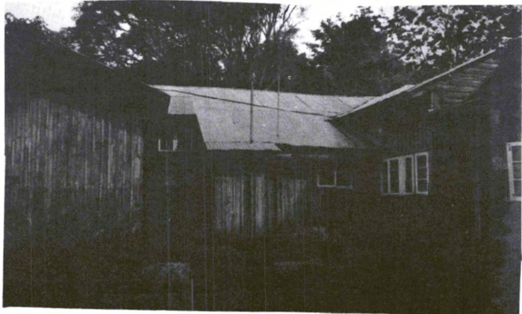
Naivasha Housemaster's House Falling To Pieces.
